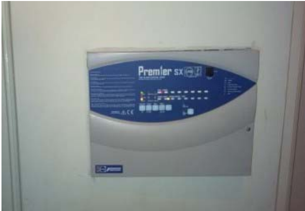
The fire alarm panel is showing a fault and in room 16 next to the faulty alarm panel we are informed a relative of Kevin Scott (Manager) is living there
