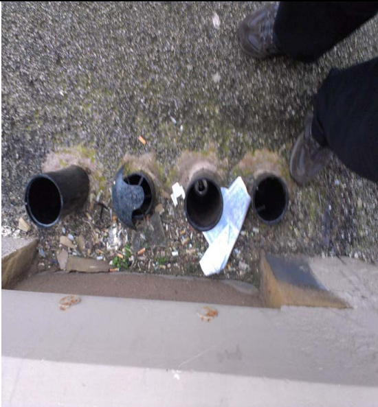
7) Incoming air and flue arrangements that are damaged blocked by cans and debris
