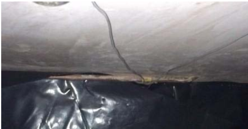
Electric cable wrapped around a copper gas pipe, if the electric cable was to be damaged it may result in the gas pipes conducting electricity leading to potential electric shocks
