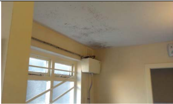
Photographs showing the damp issue in the customer toilets and evidence of a water leak from the ceiling
