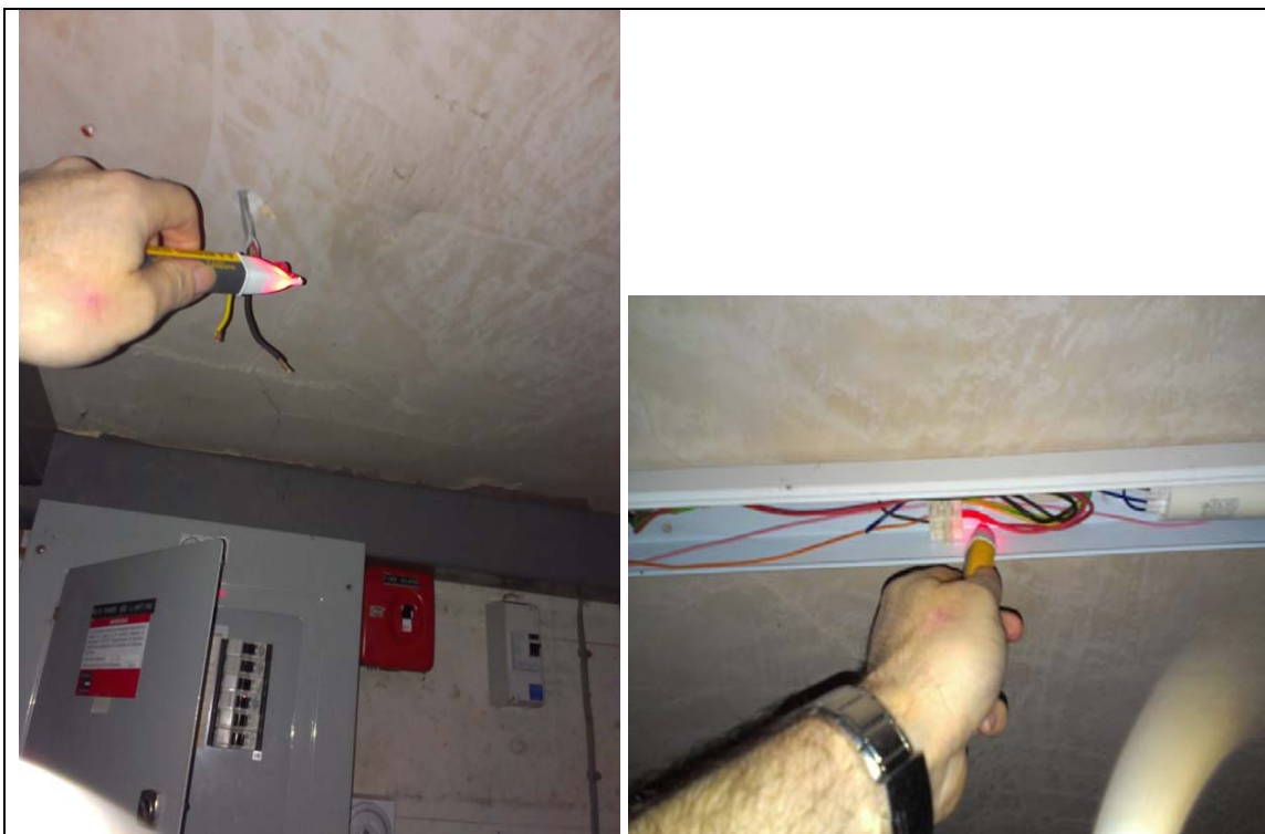
5) Live electrical conductors exposed at >200 volts.
